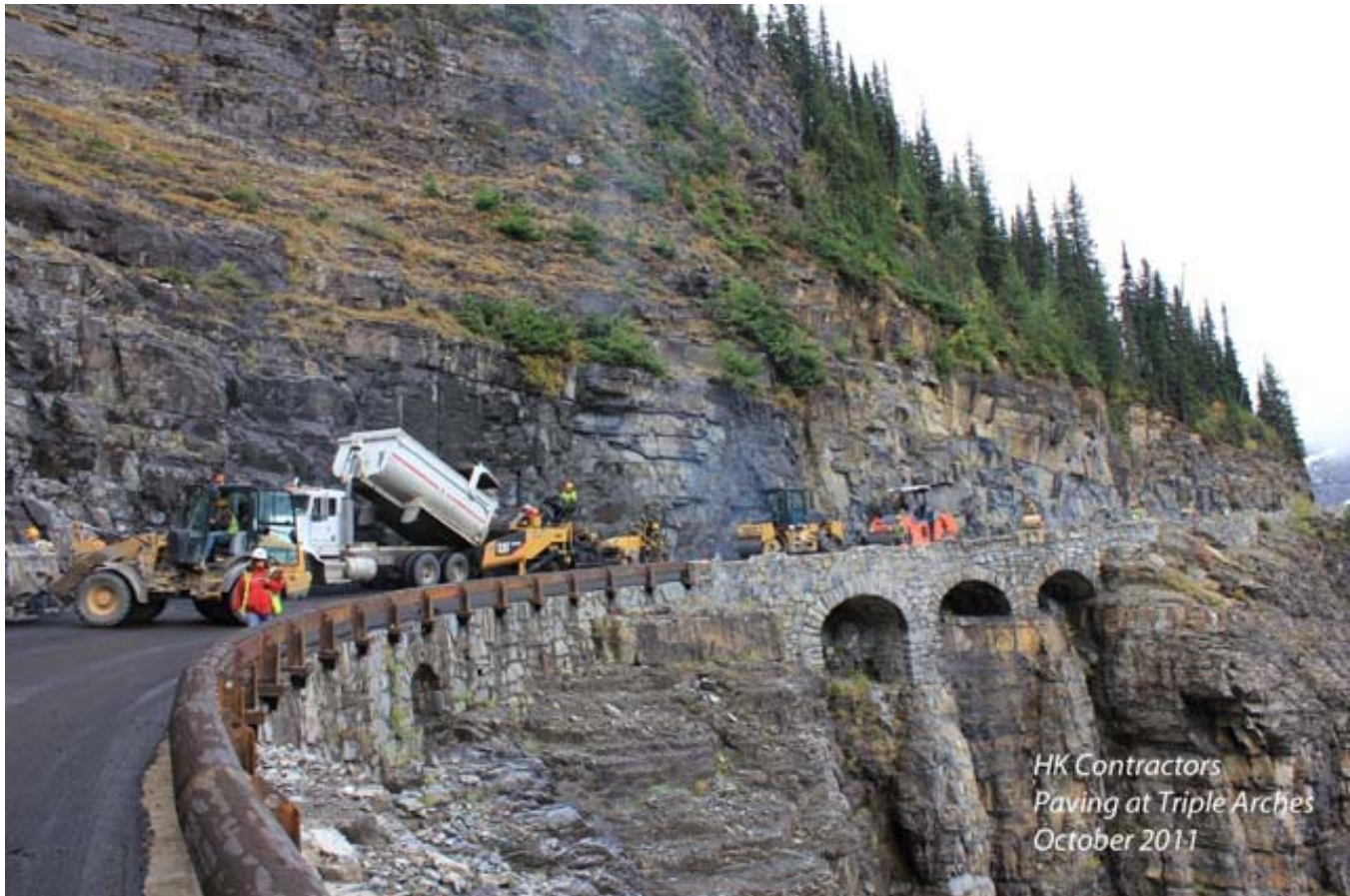
Construction personnel working on a stretch of the Going-to-the-Sun Road. (Courtesy of WFL)
