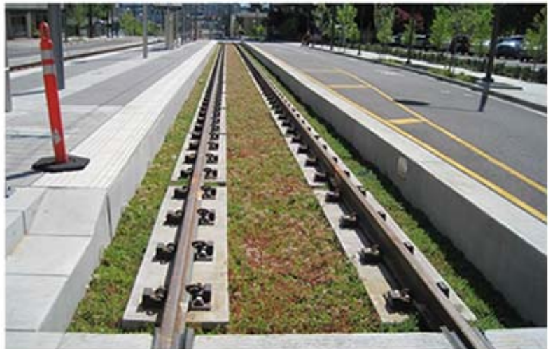
The light rail project piloted the use of “eco-track”, which employs a planted trackway instead of paving. Similar in form and function to a green roof, the sedum plants in the trackway provide runoff capture, as well as aesthetic benefits and insect habitat.
